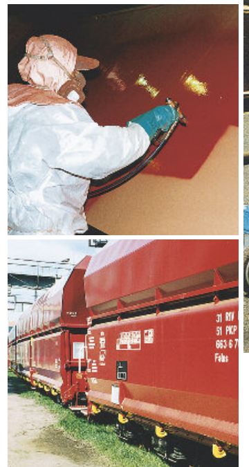
A railcar for transporting food is being coated with a solvent-free, thick polyurethane coating using a WIWA DUOMIX 333 (solids: 92,5%, potlife: 5 minutes, spraying temperature: 60°C).
