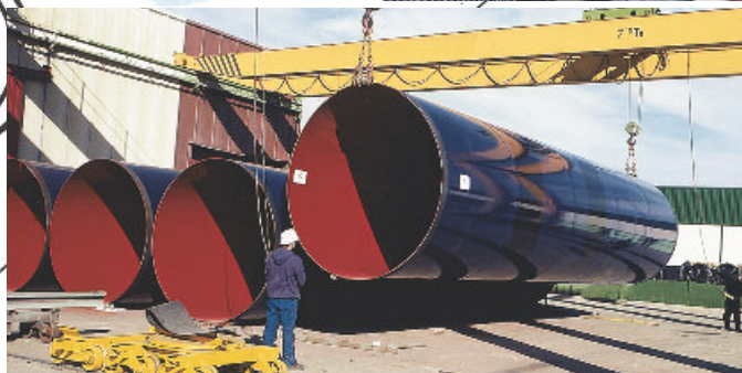
Here, pipes were sprayed with a polyurethane coating material (potlife: 30 seconds, spraying temperature: 55°C) using a WIWA DUOMIX 300.
